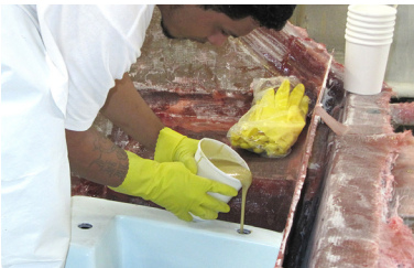
Using foam in aft hull to prevent 6011 from escaping during transom pour
